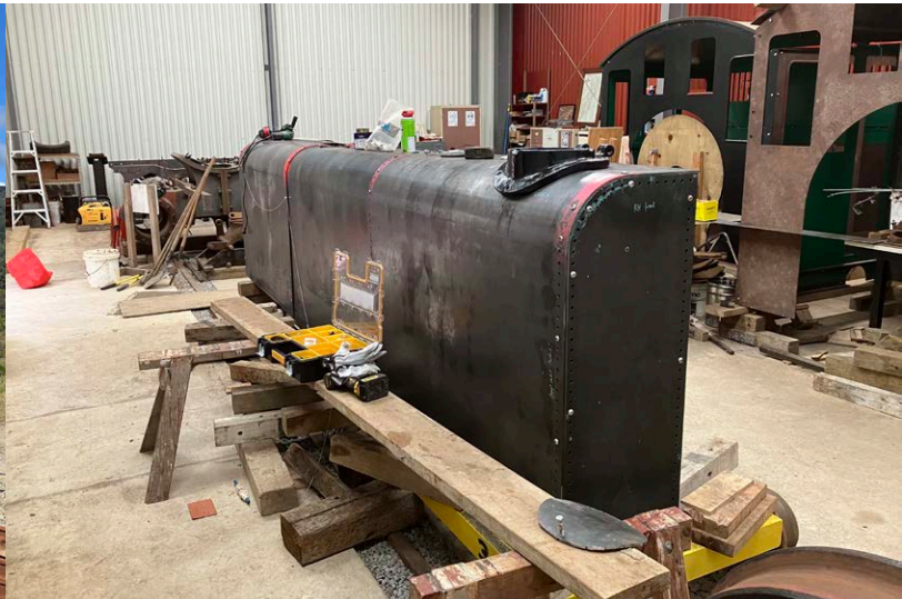
Work continues on rebuilding components of the two Wb-class Baldwin steam locomotives - Wb 292 and Wb 299. The driver's side tank's seen here inside our workshop, with original filler lid try-fitted. Cabs for both locos to the right.
