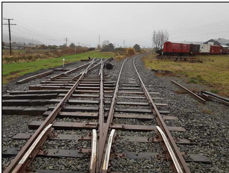
The new siding to the ballast pit: a double slip has been connected to the turnout on the back leg of the triangle and is being rebuilt. 27th June 2020. Photo: Peter Jenkinson
