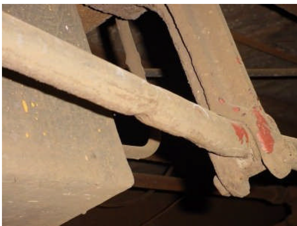
Corrosion of truss rod at battery box attachment
