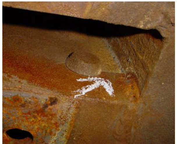
Crack propagating from rivet
