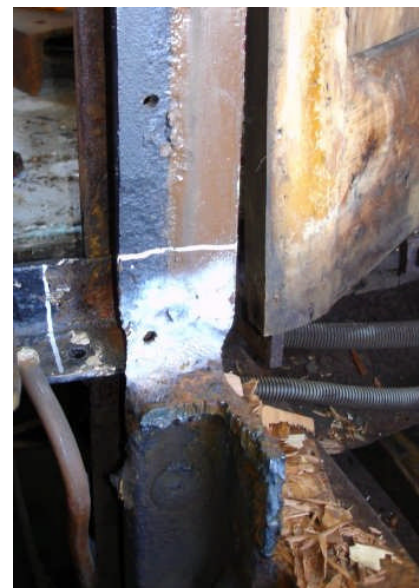
Severe corrosion at bottom of side doorpost
